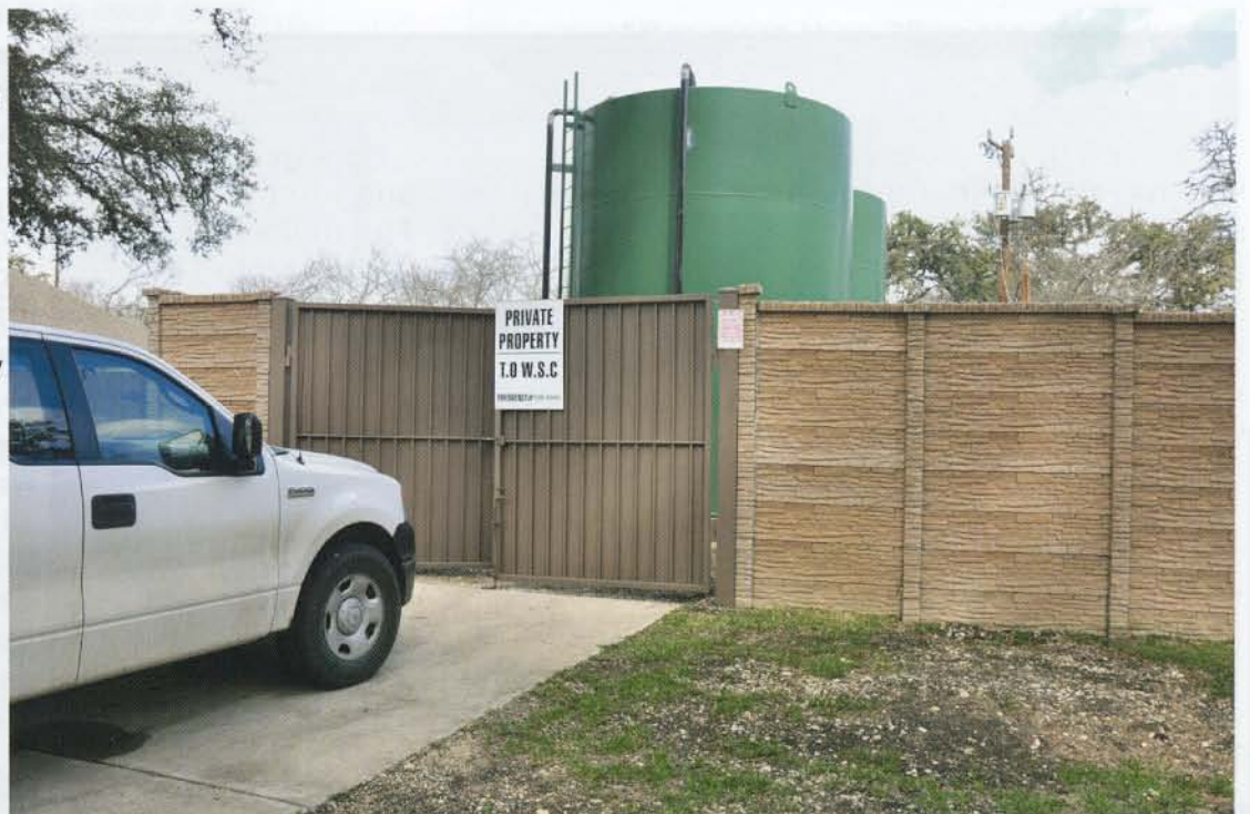
The utility replaced the old metal fencing with masonry to improve security and the appearance of utility infrastructure in the residential area.
