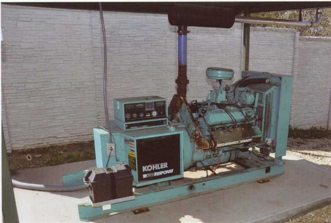
The utility purchased a back up generator to keep pumps running in the event of a prolonged power outage.
